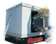
Compact Sub Stations
